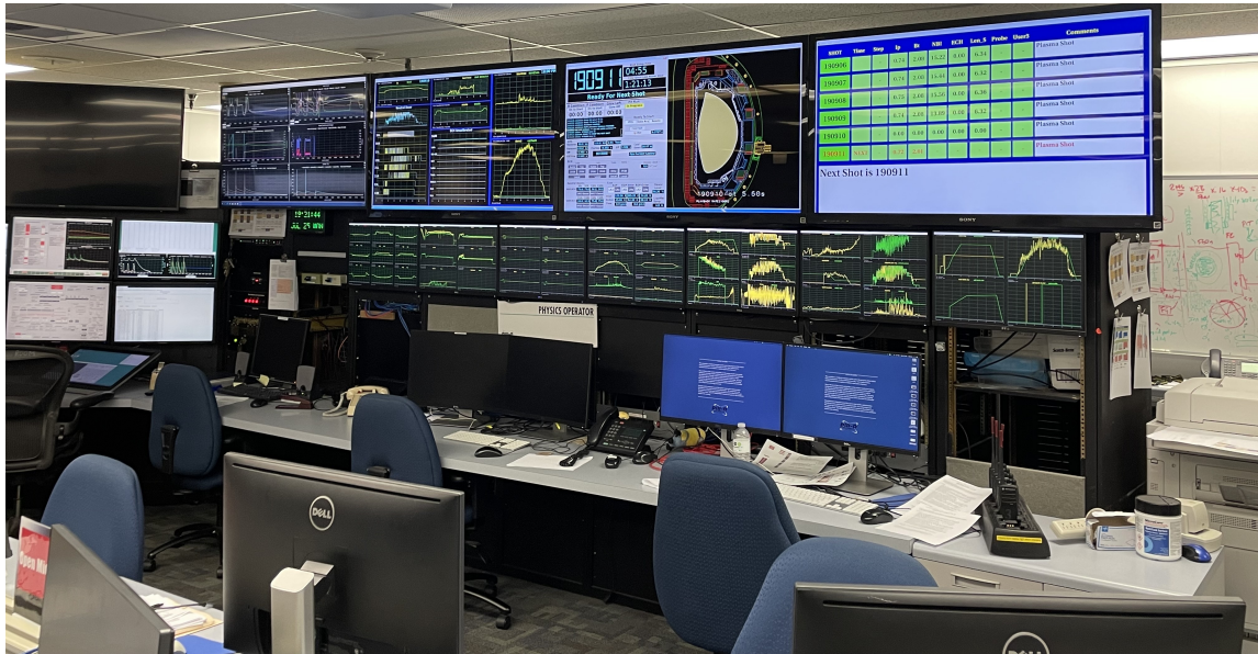
Figure 10.2: The control room at DIII-D.
